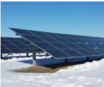
➤ Solar panels installed at Verizon facilities in Billerica, MA.
